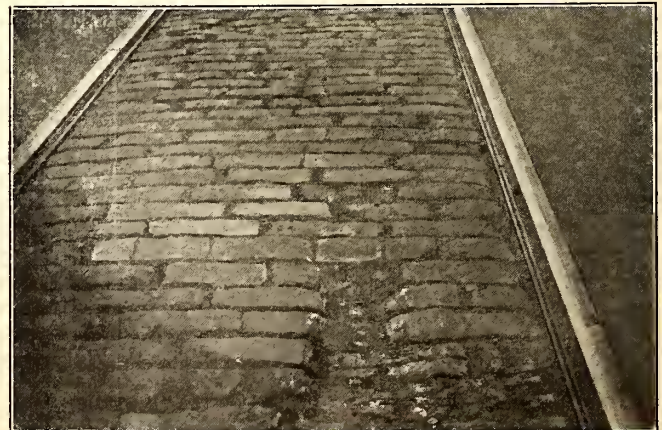
TRACK MAINTENANCE DATA—FIG. 8, GRANITE BLOCK PAVING SHOWING DAMAGE NOT CAUSED BY RAILWAY
